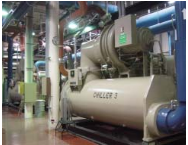
Mutual of Omaha Chiller Plant, Omaha, Nebraska
